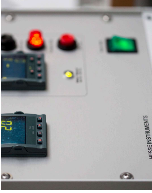
Furnace control unit
